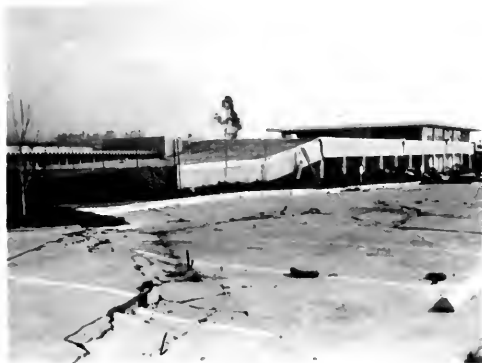
Photo 8. View northeast from front parking lot of San Fernando Juvenile Hall shows severe damage to building. It also shows northwest margin of ground cracking caused by shaking and consequent movement of ground in right part of photograph to southwest toward camera. Cracks in foreground show right-lateral displacement; those on opposite end of parking lot (off the right side of photograph) show left-lateral displacement. Photo by James E. Kahle.
